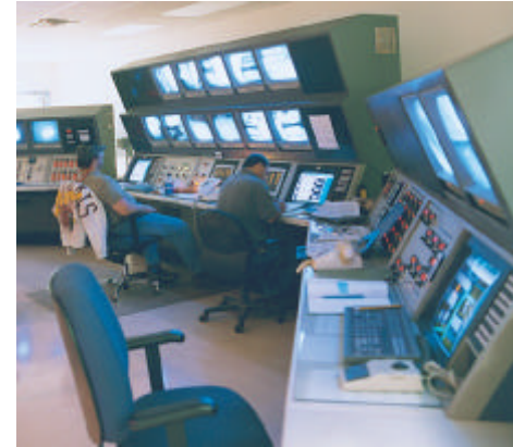
Furnace control system
