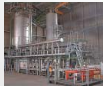
Recuperative furnace melting C-Glass and performing at 200 metric tonnes/day (220 US tons/day) at 1250 kcal/kg (4.5 MBTU/US ton)
