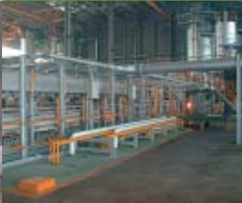
Distribution channel/forehearth system designed for 250 metric tonnes/day (275 US tons/day)
