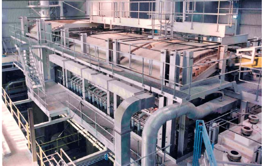
Under-port gas firing system for a new end-port furnace recently installed in the UK
